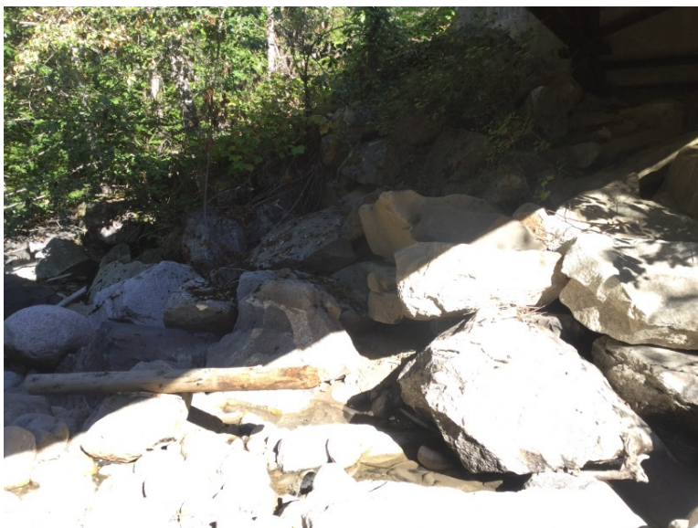
Riprap scour downstream right bank
