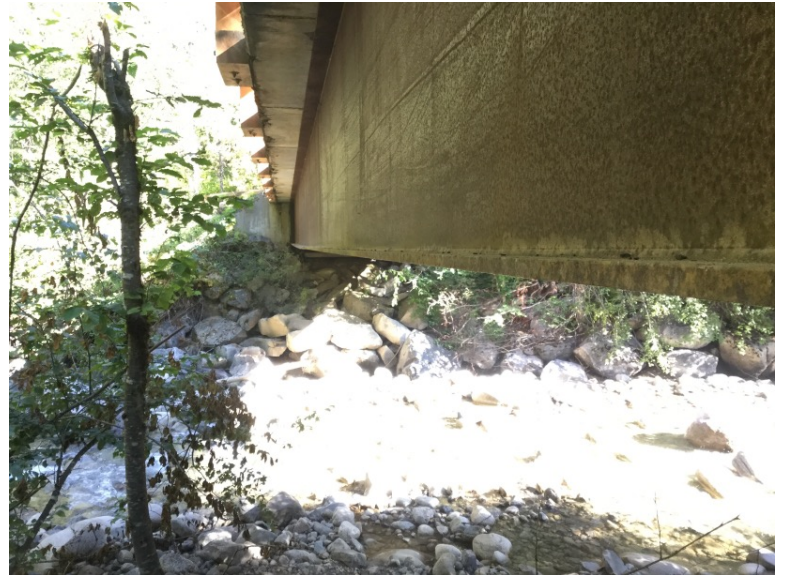
Visible sag in girders
