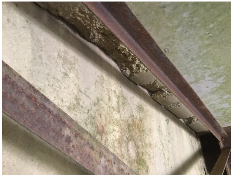
Damage under panel 1 at left bank
